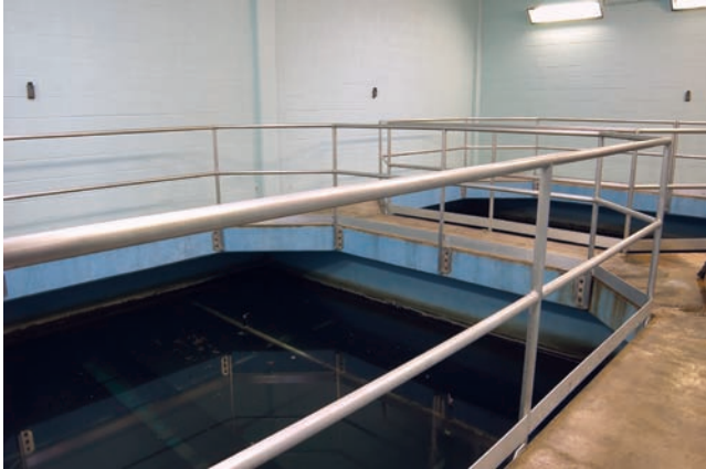
Water System Filtration Tank
